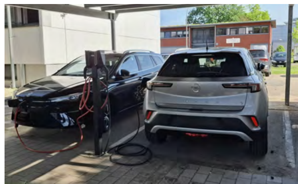
Figure 20: The FIZ Karlsruhe charging station.
