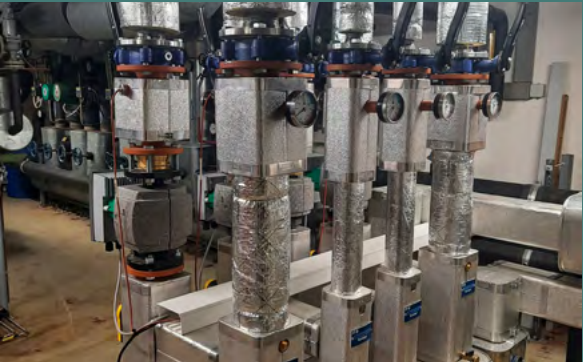
Figure 22: The new district heating transfer station for Building 240
